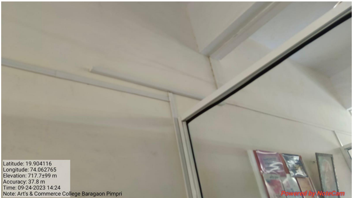
LED LIGHTS IN STAFFROOMS
