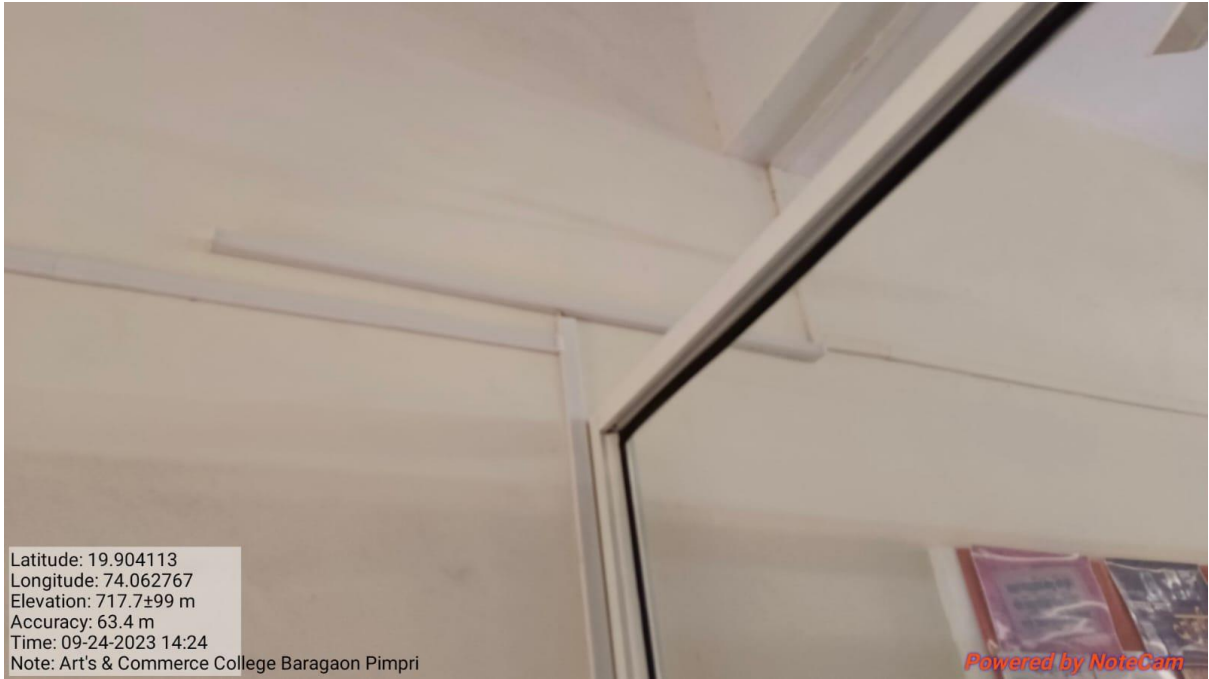
LED LIGHTS IN STAFFROOMS
